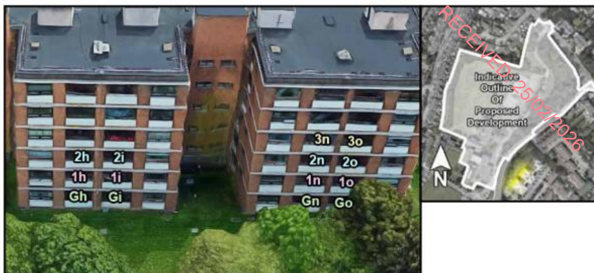
Fig. 5.4 Affected windows on Rowan Hall / Cedar Hall (L) Aerial view of assessed locations (R)
